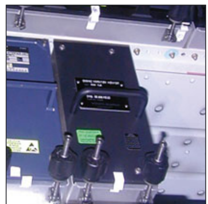
Vibro-Meter EVM in A320 electronics bay
